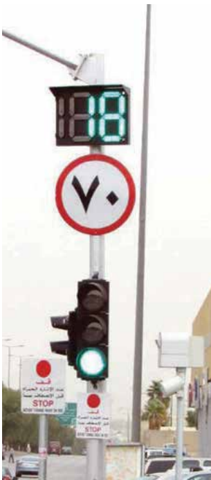
Countdown timer installed at a traffic signal in Saudi Arabia
